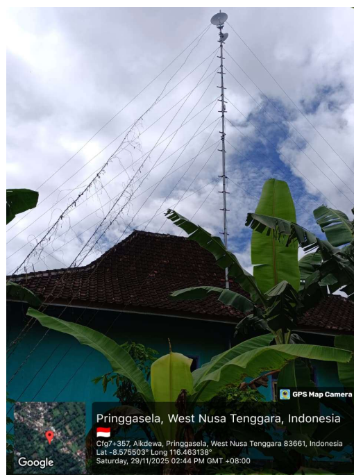
Figure 8. Signal Receiving Antenna (station 1)
